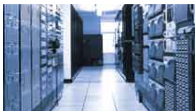
DATACENTER and IT
